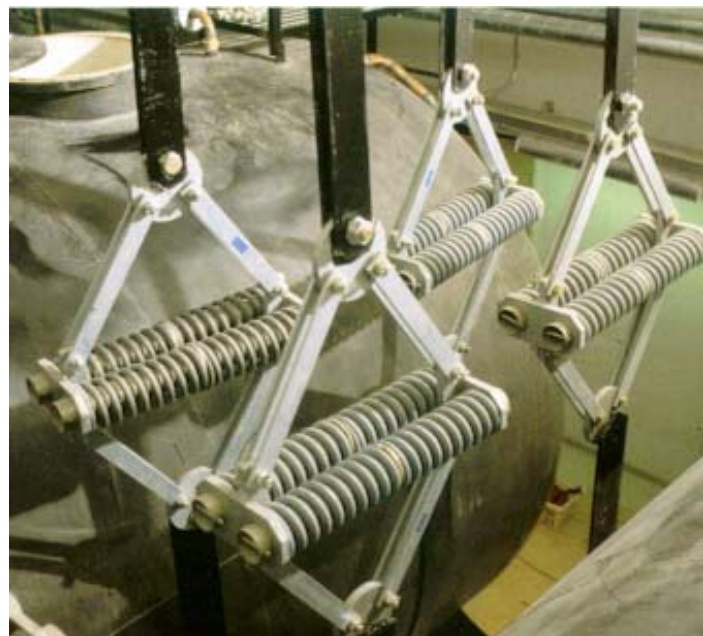
An overhead mounting of large fuel tanks with VTV2G/35-J Ground Shock Isolators
